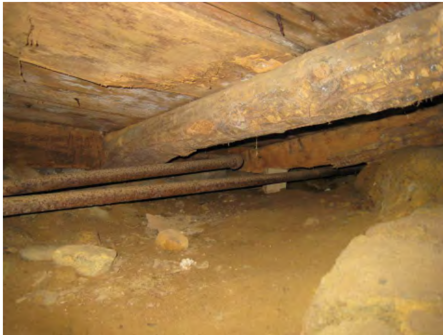
Photo 5 Collapsed first floor framing section (Facing north/Middle Road, center section north of chimney as viewed from crawlspace)
