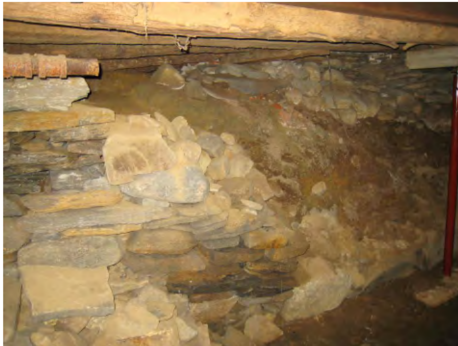
Photo 2 Failing foundation wall, west side of chimney (Facing east, toward driveway/parking area)
