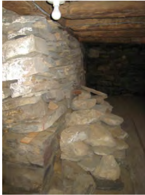
Photo 1 Failing foundation wall, east side of chimney (Facing north, toward Middle Road)
