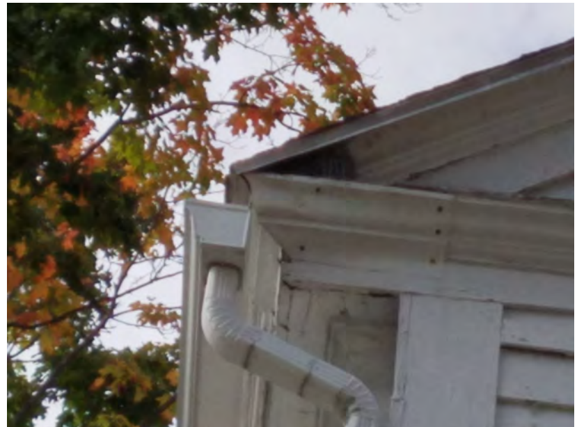
Condition at southeast cornice return. Note sheet metal repair.
