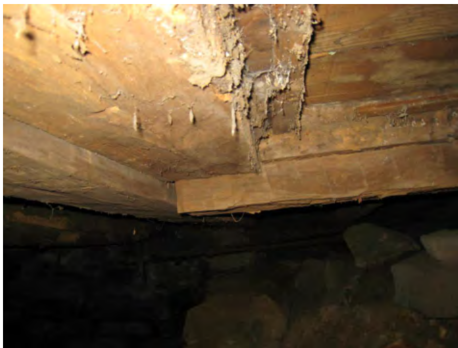
Photo 4 Beam previously supported by now-collapsed chimney wall (Facing north, toward Middle Road, showing split at mid-depth)
