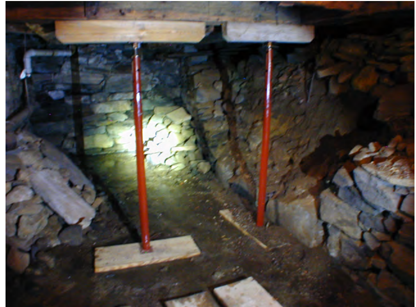
Failure of the stone foundation at the chimney.
