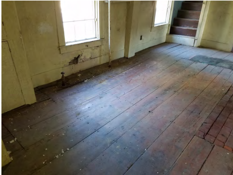
Sagging floor at north side of the Old Kitchen.
