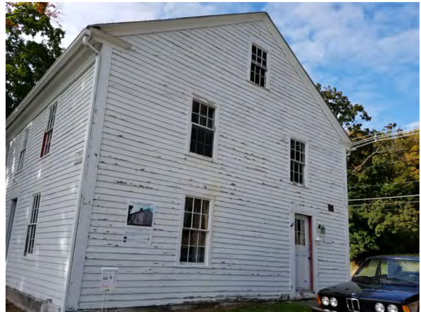
Typical condition of paint. East side shown.
