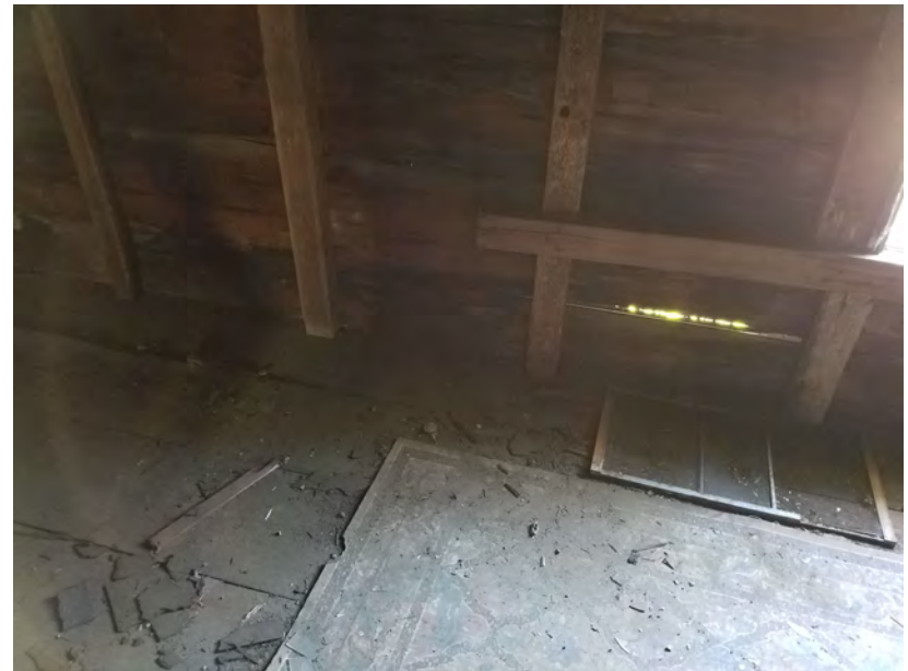
Gaps in the gable end siding and sheathing at the attic.
