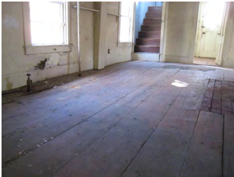
Photo 6 Collapsed first floor framing section (Facing northeast/Middle Road, center section north of chimney as viewed from first floor)
